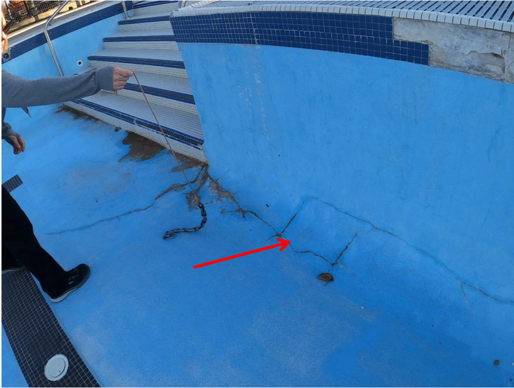
Movement at the stairs evident by cracking extending toward the deep end.
