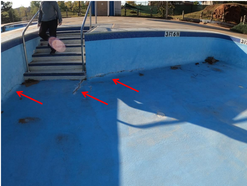
In the slide area there is movement similar to the lap area at the stairs.
