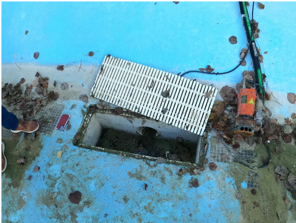
Drains are poured in place and may need to be reviewed for updated VGB requirements for SOFAs.
