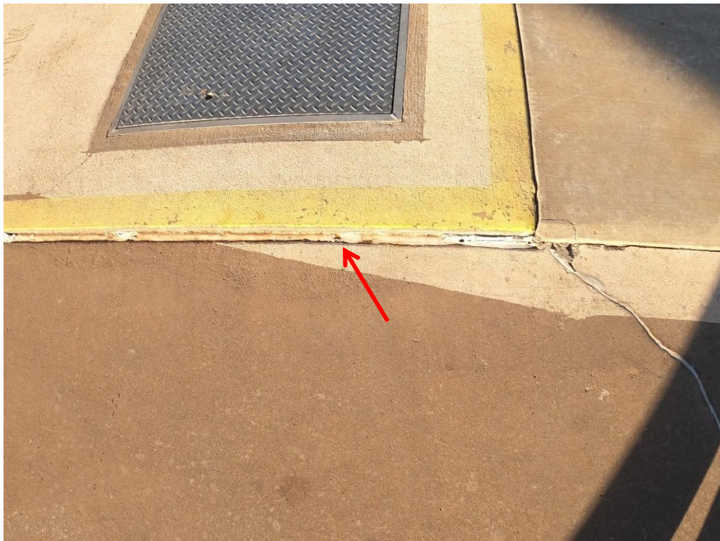
The deck around the pool surge tank has dropped and cracked. The joint sealant has failed.
