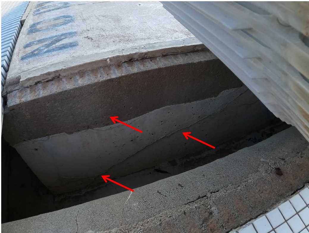
Waterproofing coating does not extend high enough on the backside of gutter. There is also cracking on the backside of the gutter.
