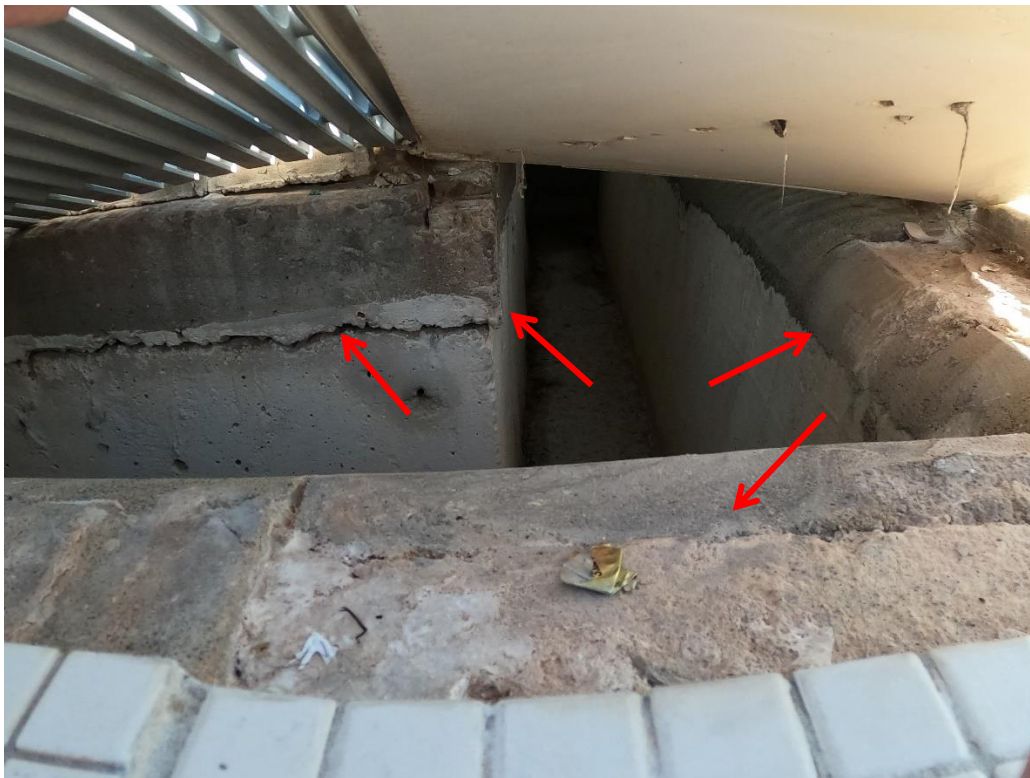
Large cold joint appears to be further separating between the deck and back wall of gutter. Waterproofing does not extend high on the back wall of the gutter.
