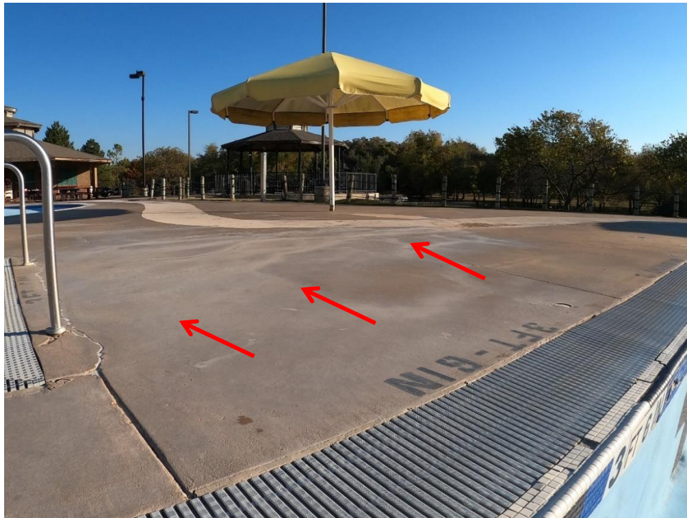
The deck north of the lap area has a low spot that appears to be stained from water ponding. The number of deck joints is insufficient to control cracking.
