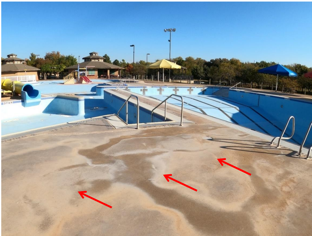
The deck south of the slide area has low spots. Water staining is apparent where water is not draining.
