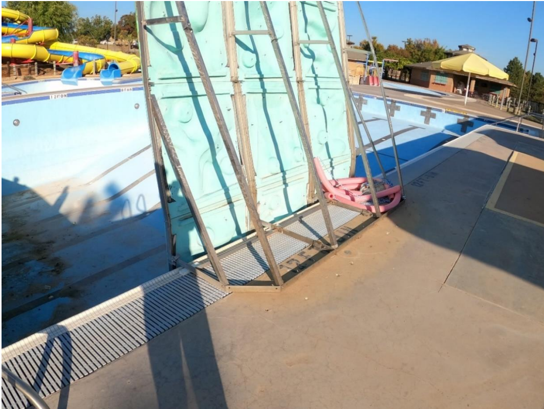
There is no bonding wire to the climbing wall and needs to be tied to the pool.
