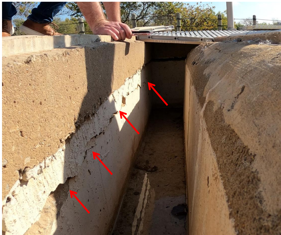
The crack begins roughly mid-length of wall and extends toward the stair in the lap area.
