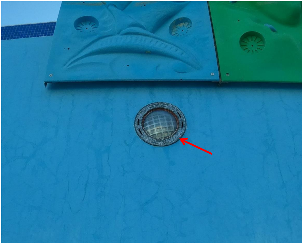
The light rings look to be corroding. It may be that the niche is not bonded.
