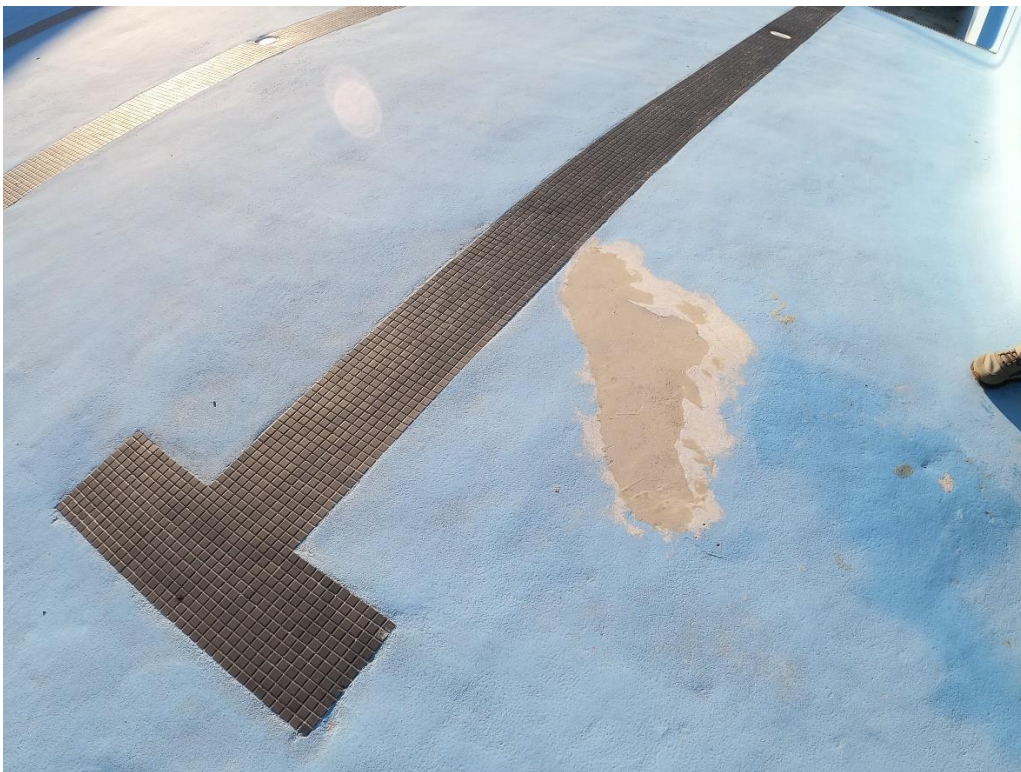
Floor patch in lap area where paint and subsurface finish has peeled off.
