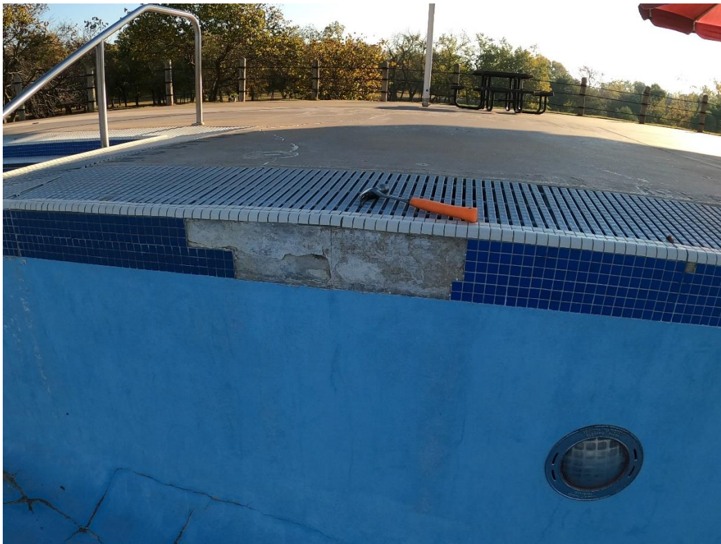
Spalling tile at gutter. Appears to have waterproofing material under the tile.
