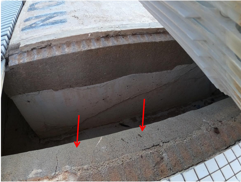
The setting or buildup forming the front gutter wall appears to be too grainy of a grout and is not coated with waterproofing on the interior.
