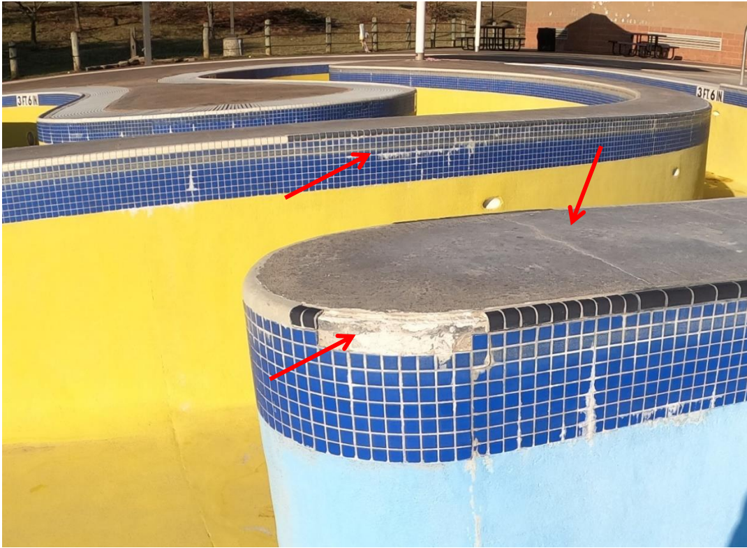
There are multiple areas of tile spalling off and cracking on top of the river wall.
