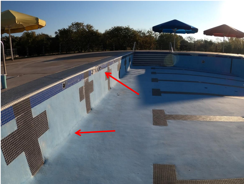
North of lap area. Cracking on base of wall and tile spalling.
